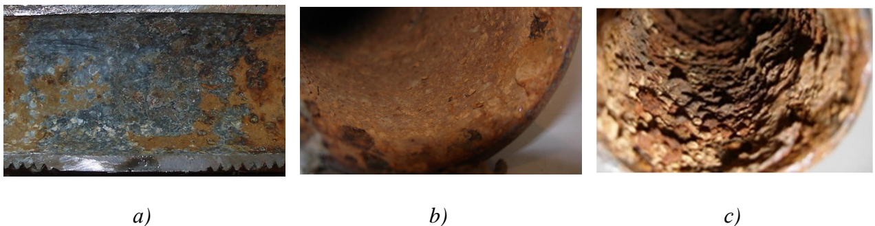
Fig. 1. Image of the inner surface of fragments of CWS Ø25 (a), CWS Ø76 (b) and HWS Ø42 (c) pipes damaged during operation.
